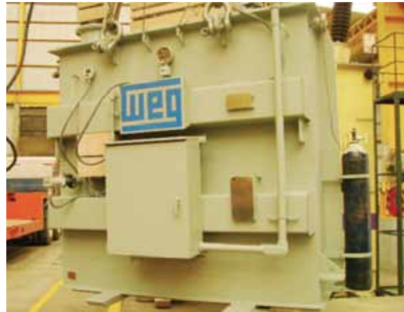
JAMAICA PUBLIC UTILITIES Jamaica 2.5 MVA – 69 kV
