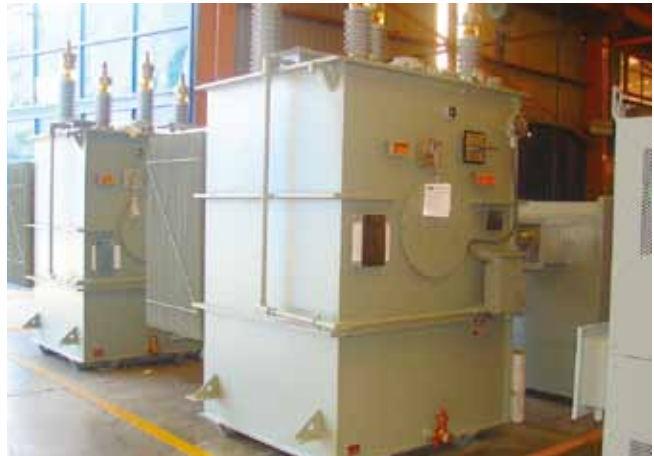
ONCOR ELECTRIC UTILITY – RICE SUBSTATION Lancaster, TX 2.5 MVA – 69kV
