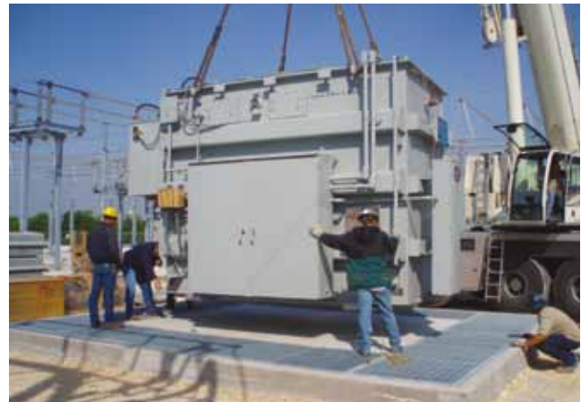
GUADALUPE VALLEY ELECTRIC COOPERATIVE Gonzales, TX 24/32/40 MVA – 138kV
