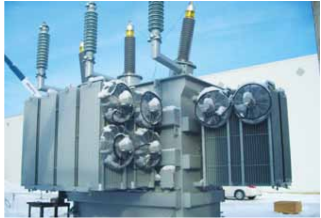
S&C DATA CENTER SUB-STATION Chicago, IL 15/20/25 MVA – 138kV
