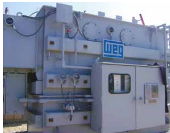
SEDGWICK COUNTY ELECTRIC COOPERATIVE Cheney, KS 25 MVA – 138 kV
