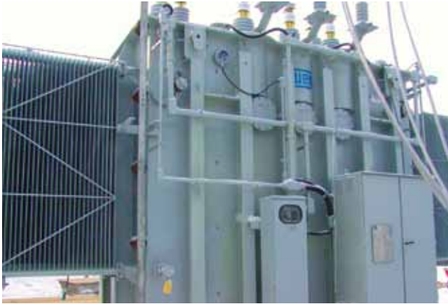
NOKIAN NATIONAL GRID Lake Saranac, NY 49.61/66.15/82.69 MVA - 115kV
