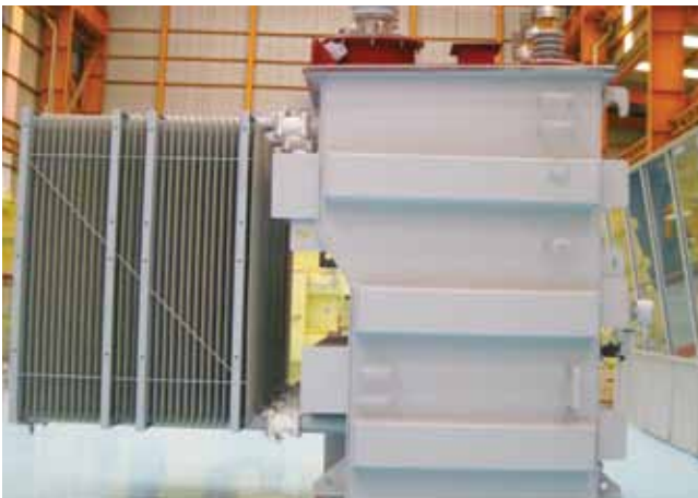
SOCORRO ELECTRIC COOPERATIVE Socorro, NM 10/12.5 MVA – 115kV
