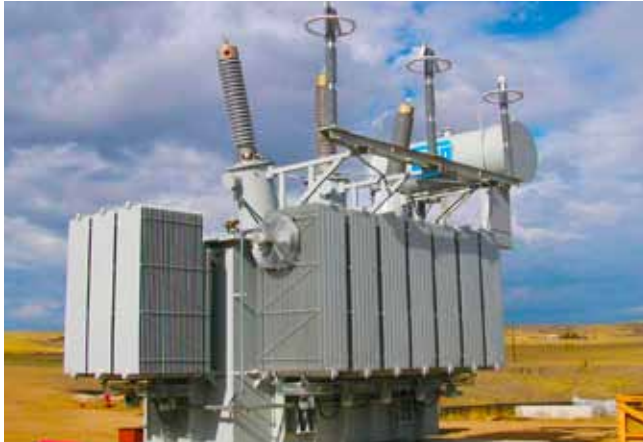
SOLAR TURBINES Butte, MN 75 MVA - 169 kV
