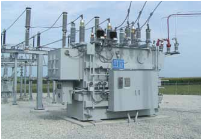
LOUP RIVER PPD Genoa, NE 15/20/25 MVA – 115kV
