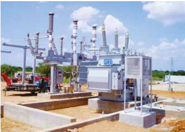
ROLLING HILLS BOOSTER PUMP STATION Ft Worth, TX 7.5/10/12.5 MVA – 138kV
