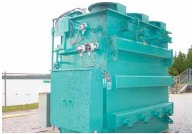
CITY OF TALLHASSEE Tallahassee, FL 7.5 MVA - 69 kV
