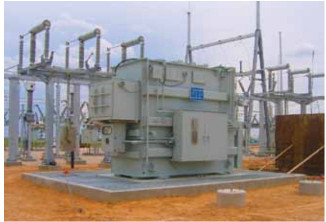
NATIONAL ENRICHMENT FACILITY Eunice, NM 24/32/40/44 MVA – 115kV
