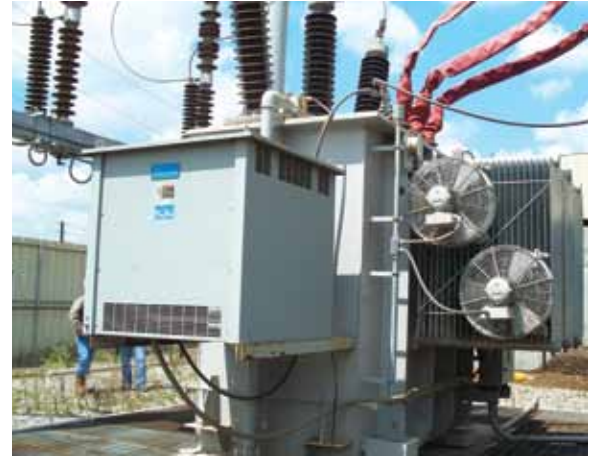
NEWELL RECYCLING East Point, GA 9.375 MVA – 145kV
