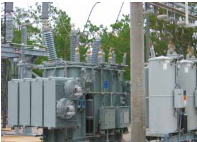
EGLIN AIR FORCE BASE Eglin, FL 10/12.5 MVA – 115kV
