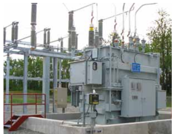
MATANUSKA ELECTRIC ASSOCIATION Palmer, AK 12/16/20 MVA – 115kV
